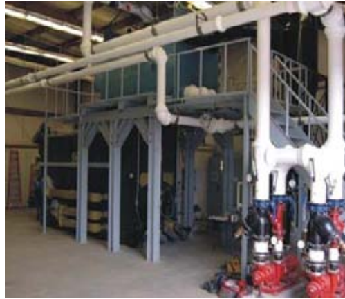
The boiler assembly with the boiler above the furnace.
