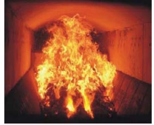
Inside the boiler where the biomass is burned.
